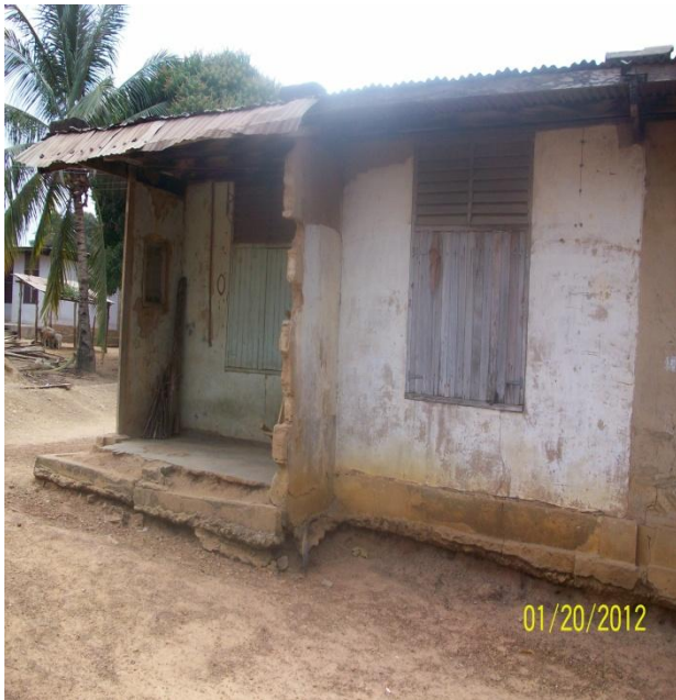
a. Resettlement house dilapidated
