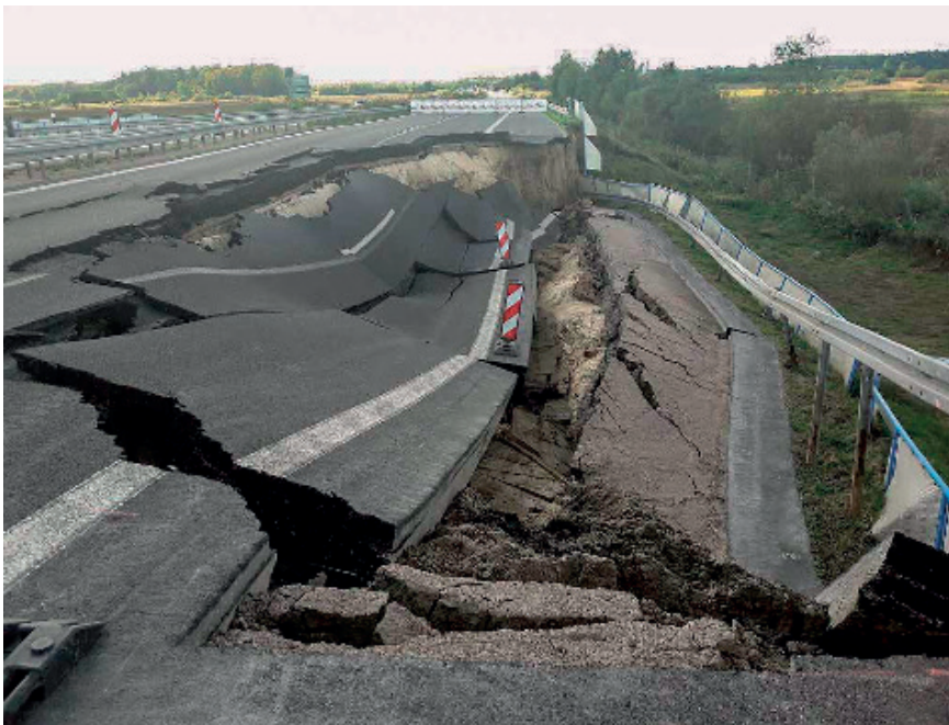
Bearing failure at the A20 Trebel-crossing in 2017. Photo by Böhme, H and Lindenau J. (2018).
