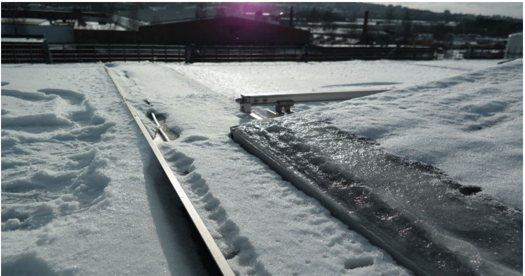
Fig. 5. An ice cap formed on the lower edge of the modules that were facing the wind. The heated gutter can be seen under the module, stretching towards the edge of the roof
