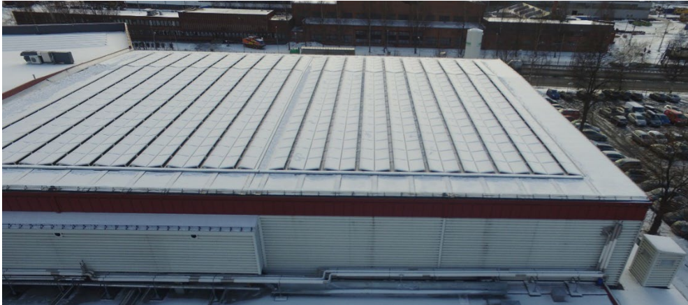
Figure 2. A typical PV snow mitigation system installed on a warehouse roof in Oslo. The system was designed by Innos (2022).
