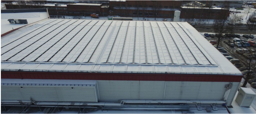
Figure 1. A photovoltaic snow mitigation system installed at a warehouse in Oslo, Norway. The modules have a low angle tilt and face each other. Between the modules are heated gutters to transport meltwater off the roof. The system is designed by Innos AS (Innos, 2022).
