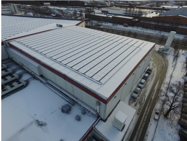
Figure 1. A PV snow mitigation system installed on a warehouse in Oslo. The system is designed by Innos (Innos, 2022).
