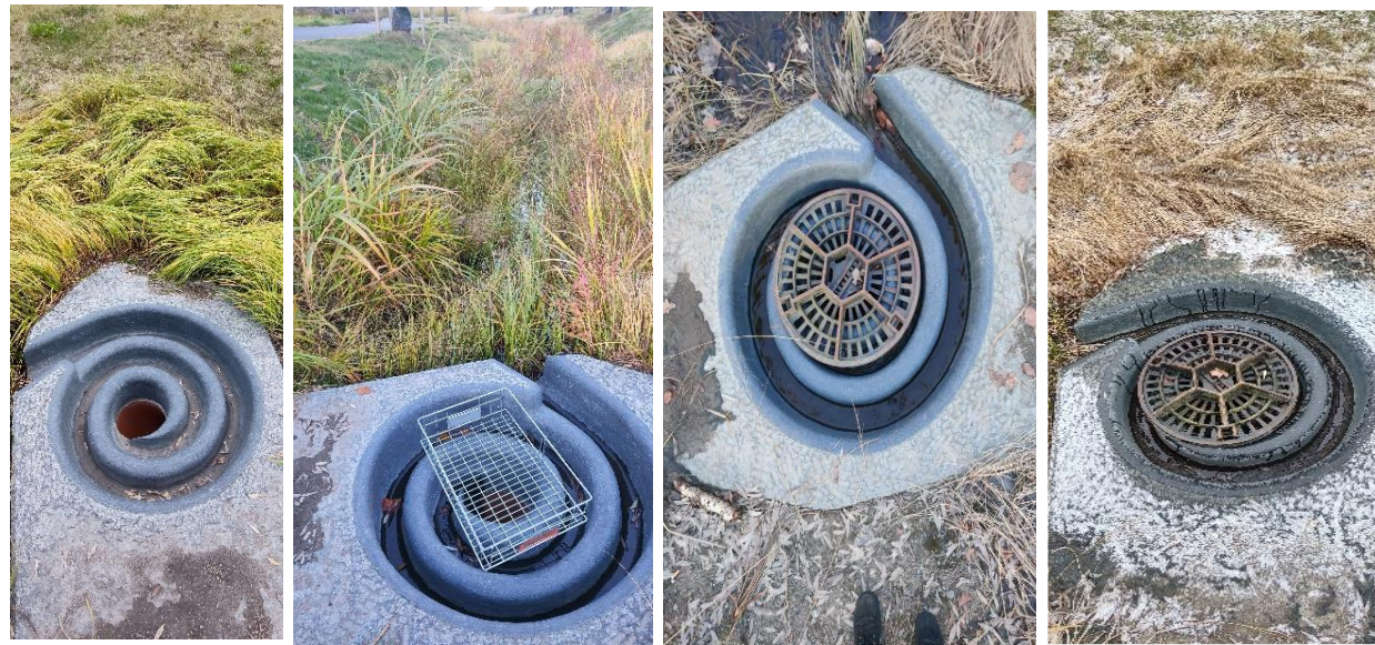
Figur 40 Photo series of evolution of a spiral designed manhole
