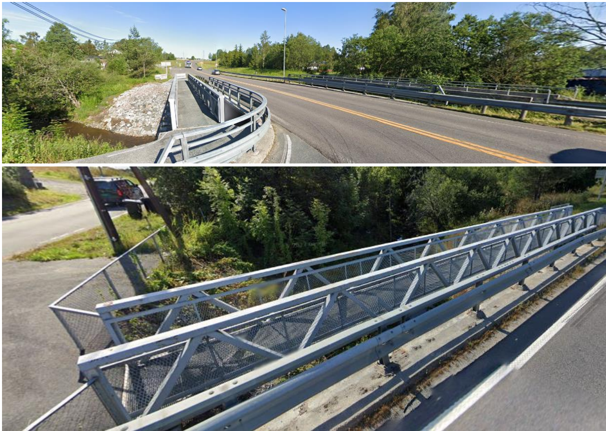
Figure 3.3: Photographs of the bridge on the left side of the road (top) and the span of the bridge crossing the river (bottom).
