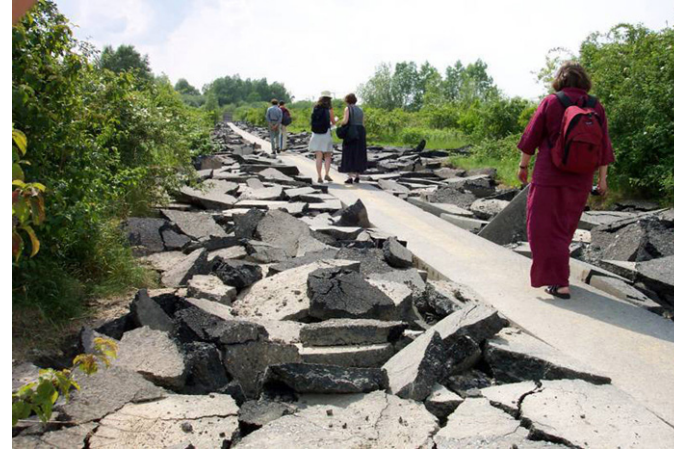
Figure 52. Cracked asphalt at the old taxiway, 2004. (Photo: Borades, D. B.)
