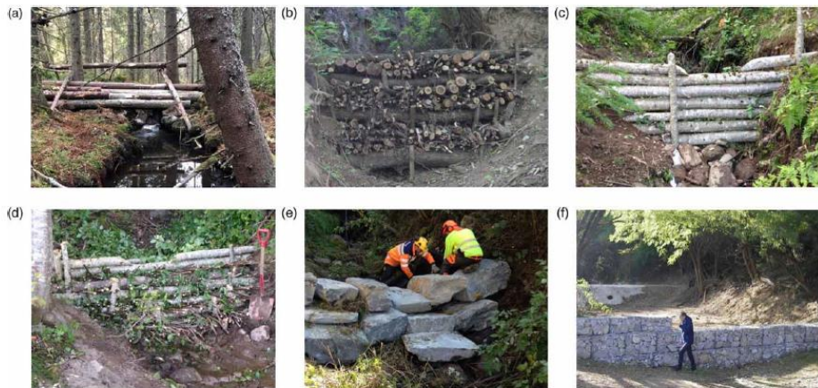
Figure 1 | Examples of online Natural Flood Detention Facilities including (a) leaky woody dam, (b) brushwood dam, (c) log dam, (d) log and branch dam (d), (e) stone check dam, (f) gabion dam. Dams a, c, d and e are made in Norway, b and f in Slovakia. Photo (e): S. Myrabo.
