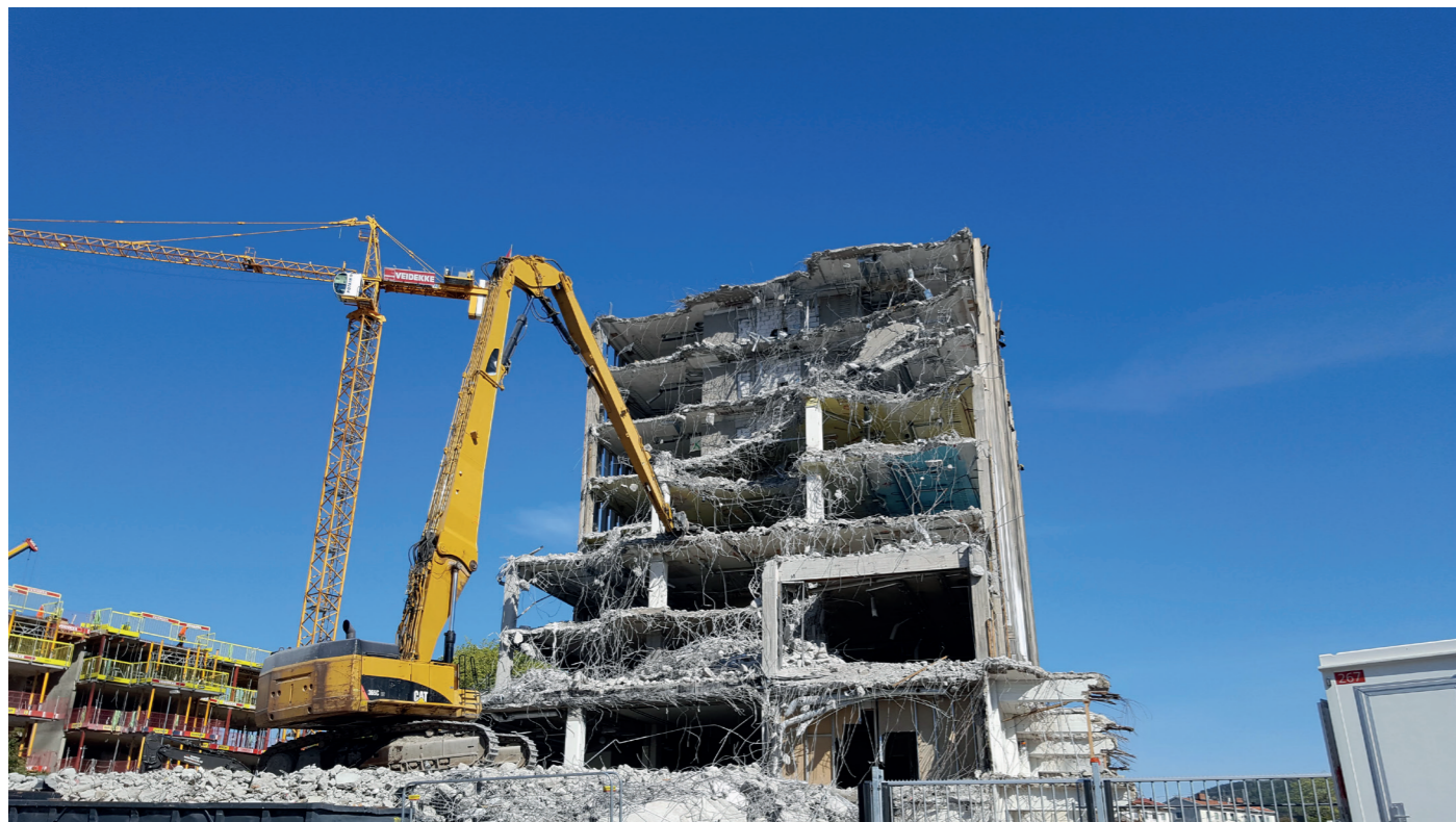
Figure 11. Demolishing concrete structures. Steel reinforcements are visible. Photo: Lasse Kilvær, Courtesy of Resirqel. 2019
