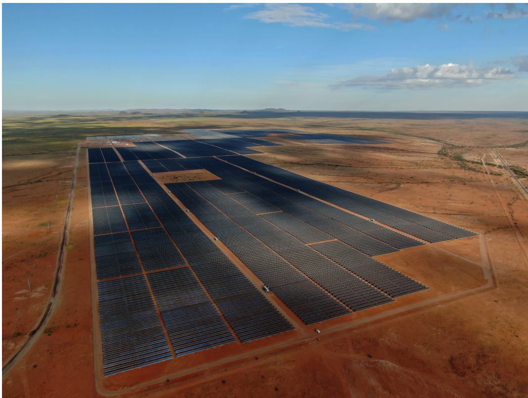
Figure 2.7: A utility-scale PV plant in the southern hemisphere.
