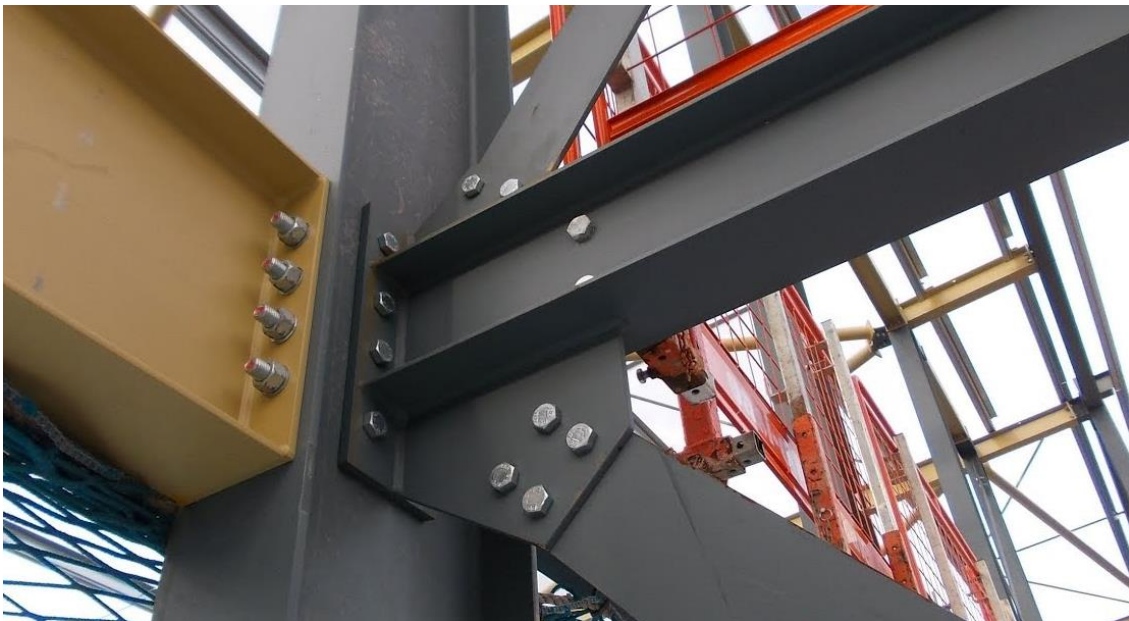
Figure 20 - Example of a bolted connection in a steel frame structure (VMC Structural, u.d.)
