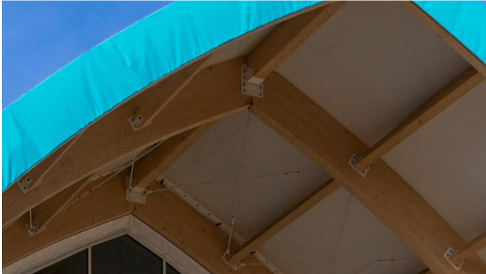
Figure 36 - Illustration showing bolted connections in the structure (photo credit: Tove Lauluten, Oslo KF)
