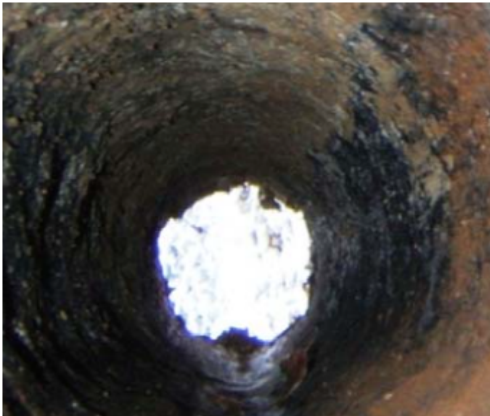
Figure 10.5: Erosion of the pipe due to sliding bed conditions (Copeland, 2013)
