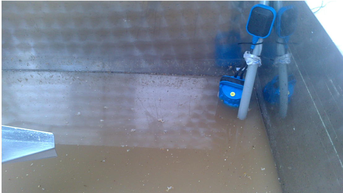
Figure 12.14: Distribution pump (Source: the author)
