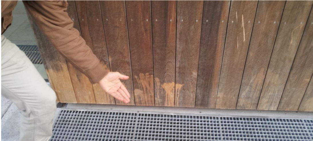
Figure 0 Wooden cladding, northwest facing wall, Astrup Fearnley Museet. Dog pee has resulted in a “clean” look compared to the darker, mouldy wood.
