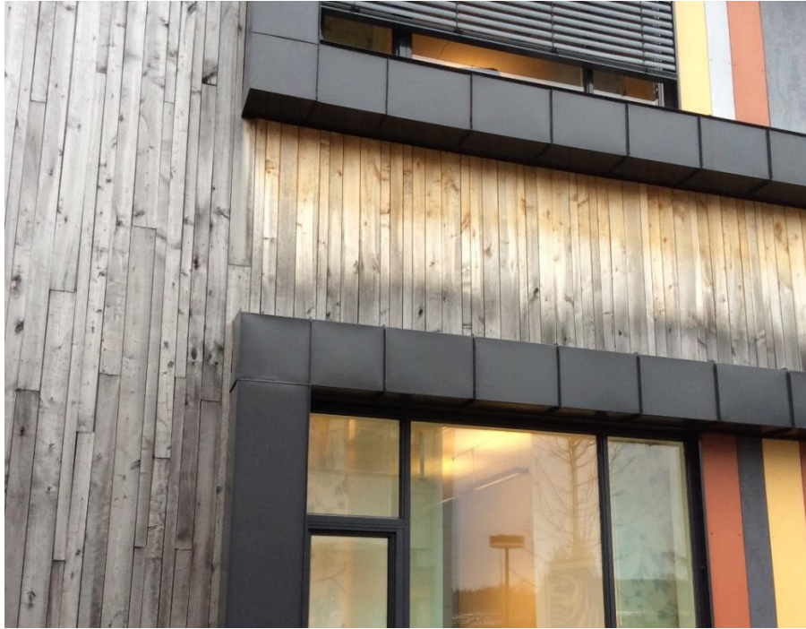
Figure 6 Ås high school. Less mould growth under the overhang.
