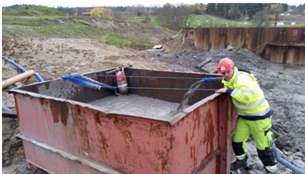
Figure 9: Steel dumpster of which the drilling fluid was collected. Person for scale (Photo: Lene Sørli Heier 2014).
