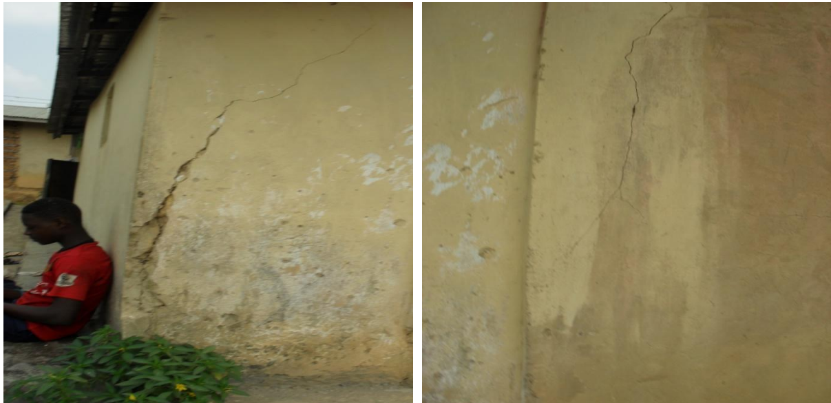
Fig. 2: Some cracked walls claimed to be due to blasting
