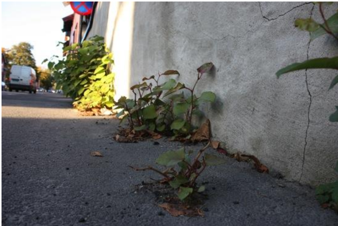
Figure 14 F. japonica spreads from the other side of the wall, and damages the asphalt layer in a street in Moss. Picture taken in September, 2013. Photo: Anne-Kari Holm.
