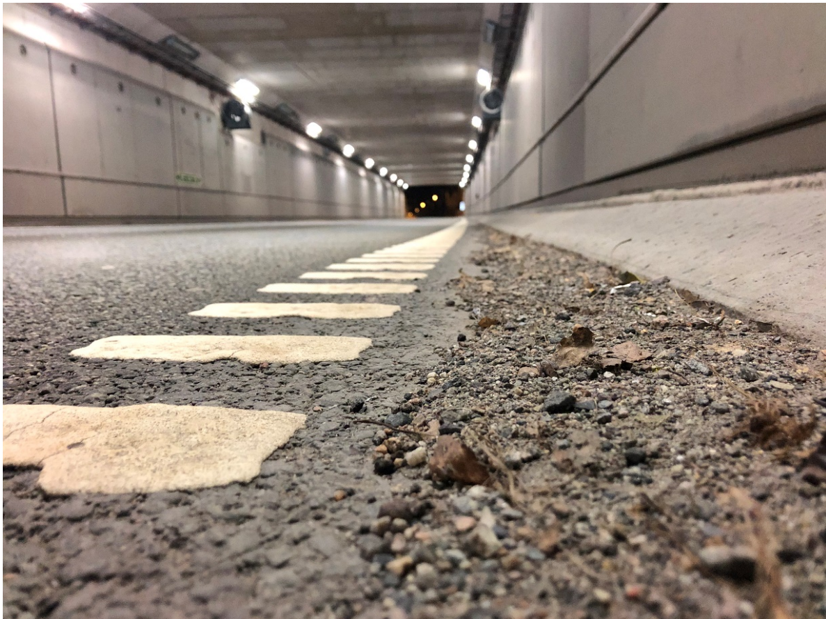
Figure 3. Example of road dust accumulating on the roadsides of a tunnel, illustrating the need for periodic road cleaning (Photo: E. Rødland)
