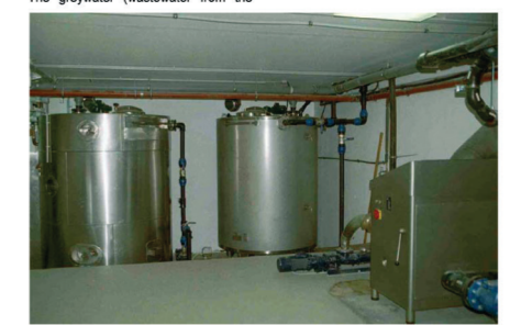
Figure 6: Mixing and neutralisation unit (source: Otterwasser)
