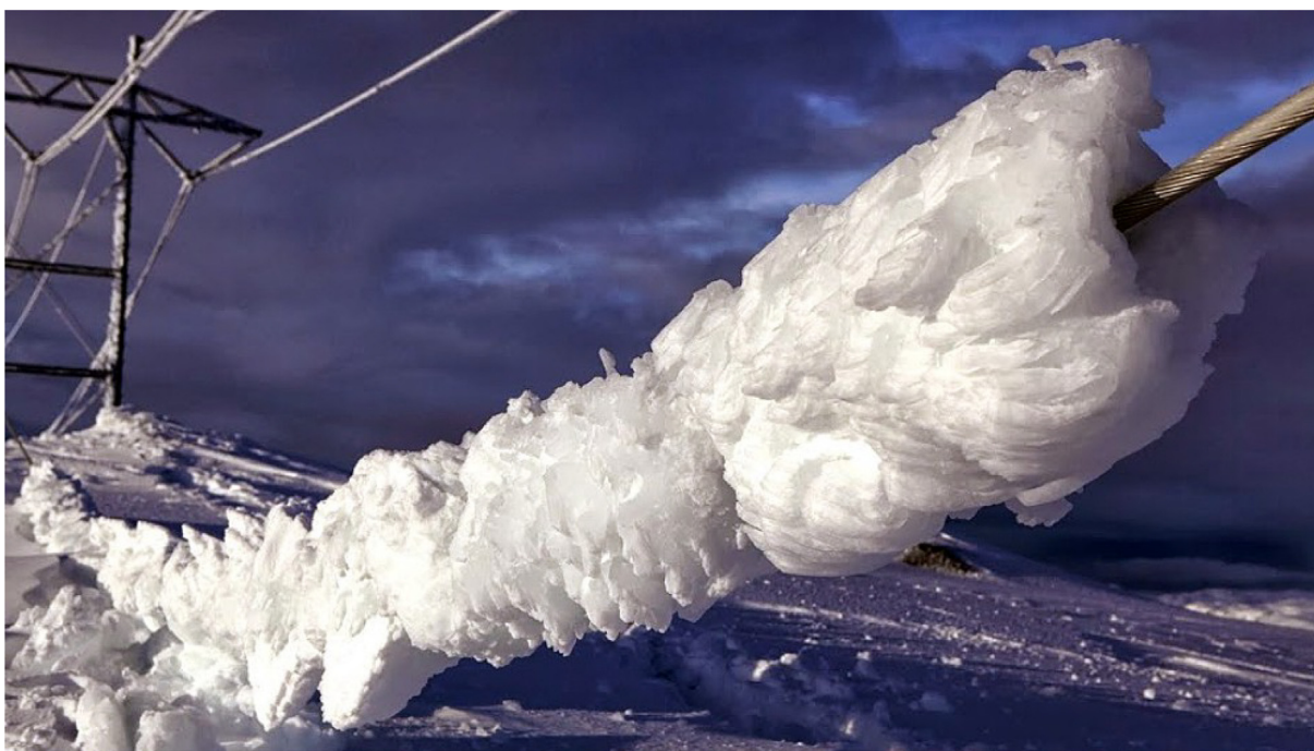
Fig. 1. Collapsed transmission line at Ålvikfjellet in January 2014. The ice loads were measured to 68 kg/m. Photo: Ole Gustav Berg, Statnett.
