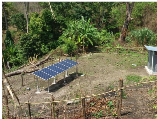
Picture 3: Solar panels for the Hoi Nam Yen water pump
