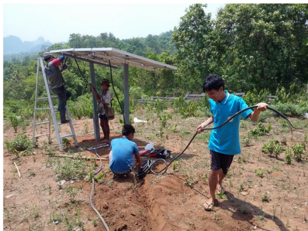
Picture 19: Kah Lah Hai students and staff helping install solar panels and wiring
