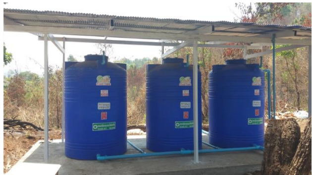
Picture 5: 2,000 liter water storage tanks in Hoi Nam Yen
