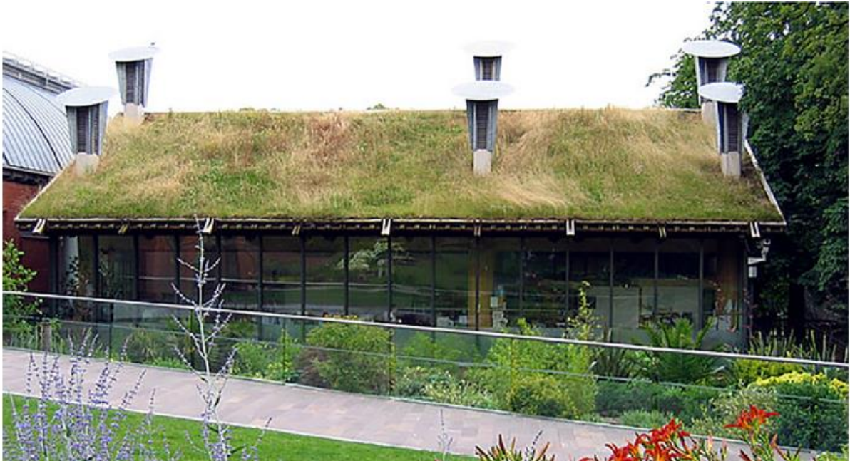
Figure 13. Green roof installed at the Horniman Museum in London (Boano et al., 2019).
