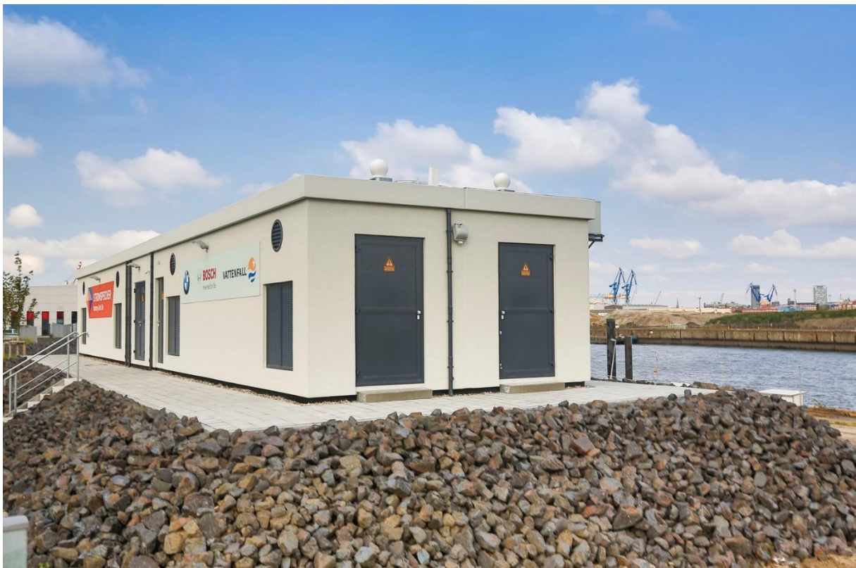
Figure 3.13: The BMW/Vattenfall/Bosch storage facility, located in Hamburg, is made up of over 100 BEV batteries, with a capacity of 2800 kWh and a power output of 2 MW. It is used for frequency regulation. Image acquired from [100].
