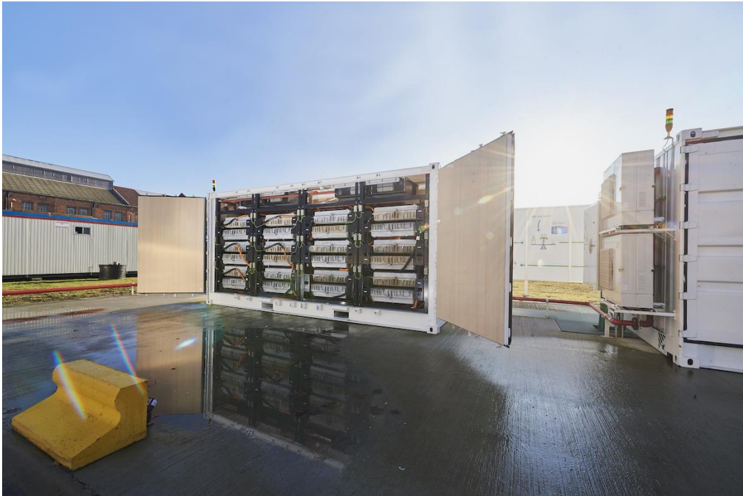
Figure 3.12: A 1200 kW/720 kWh battery system providing reactive power and frequency regulation services to the grid at Umicore industrial site in Belgium. Image obtained from [99].
