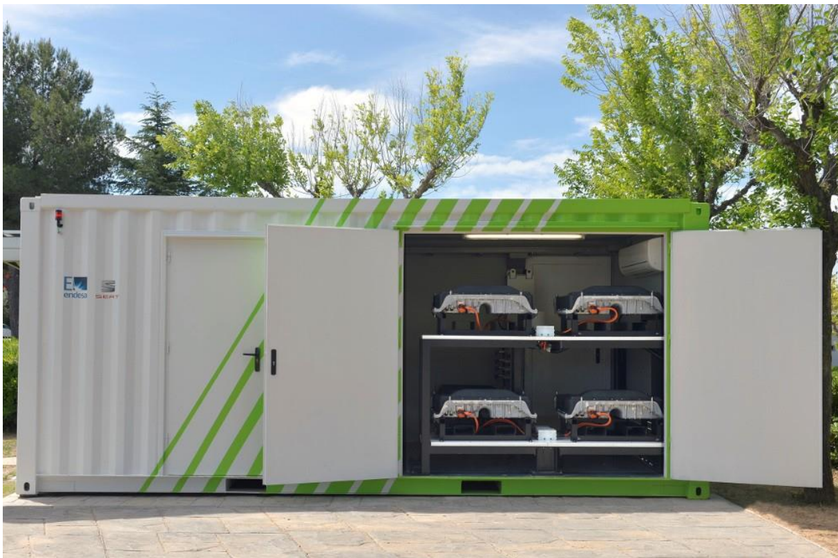
Figure 3.14: The SUNBATT living lab. Four used PHEV batteries are visible in the 15 m 2 container. The lab is also connected to a solar array, three EV-chargers, and the distribution grid. Image obtained from [101].
