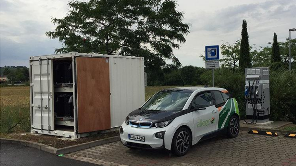
Figure 3.11: A 60 kW/90 kWh E-STOR system used as a load management system at an EV-charge site in Belgium. Image obtained from Connected Energy.
