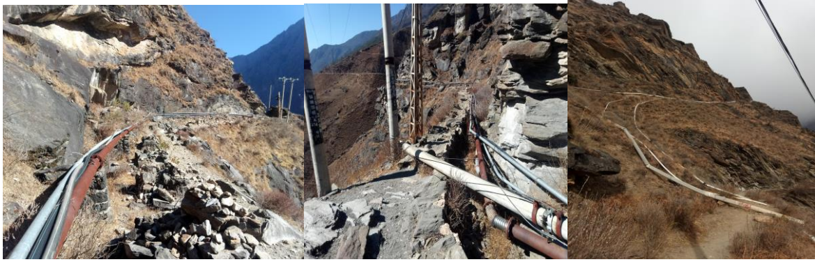
Figure 21 Pipes on the hiking trail
