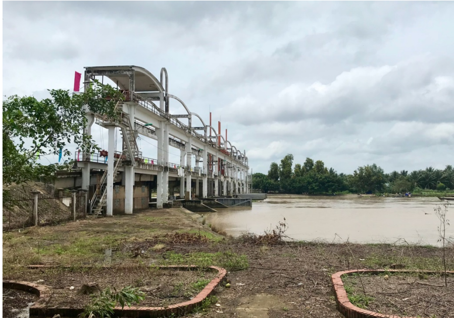
Photo 2. A gate preventing seawater to intrude the district of Tieu Can in dry seasons. Many people live outside the high-dyke (Erlend Olafsrud, 2019).
