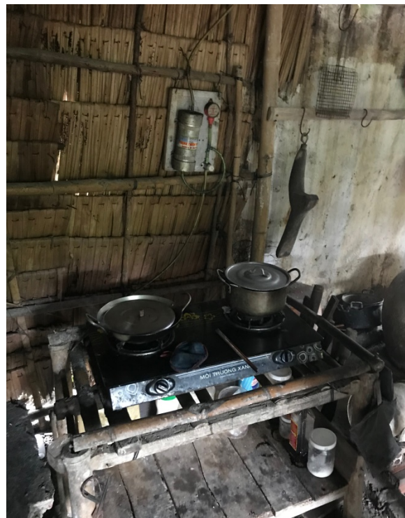
Photo 5. Biogas from pigs is brought to an indoor stove through the pipe on the wall (Erlend Olafsrud, 2019).
