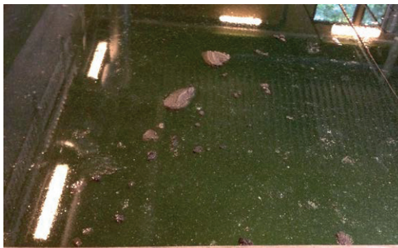
Figure 17. Failure of the sedimentation process – floating sludge
