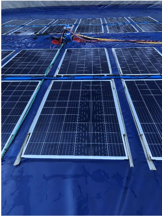
Figure 18: Solar modules on the floating canvas with a pump located between the strings.
