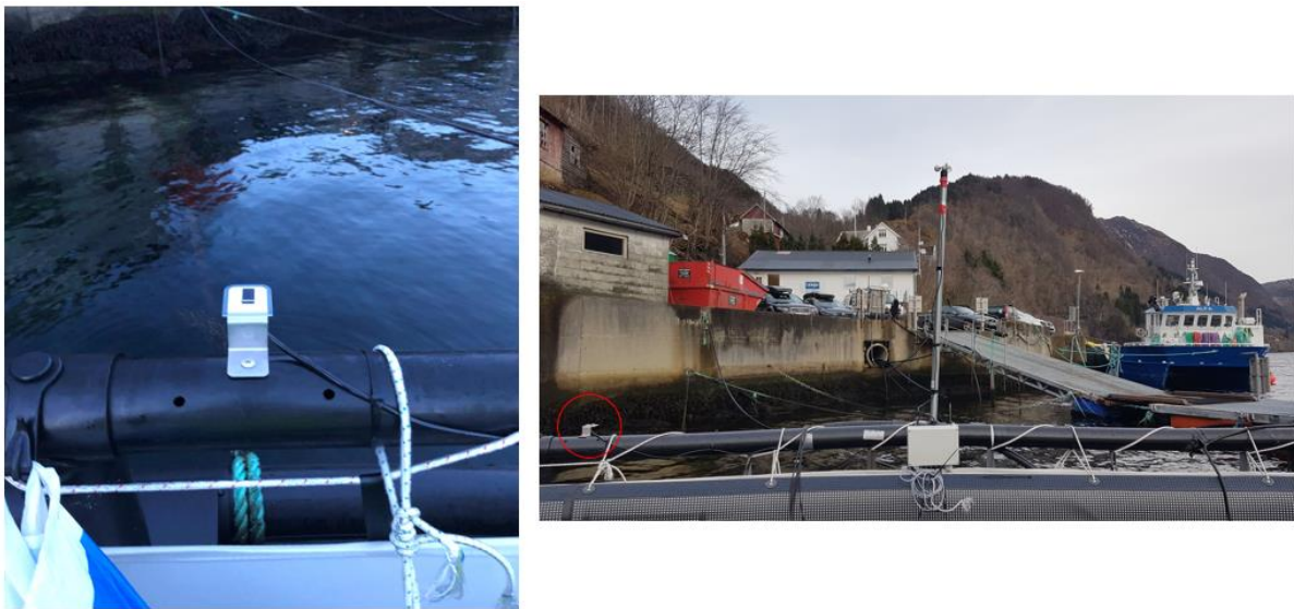
Figure 30: Left: The irradiation sensor mounted on the rail. Right: The Fronius sensor box, wind speed instrument and irradiation sensor to the left.
