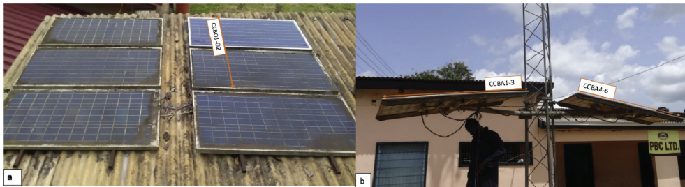
Fig. 3 – Pictures of installations: (a) Battery-charging installation at Akim Oda and (b) Battery-charging installation at Breman Asikuma.
