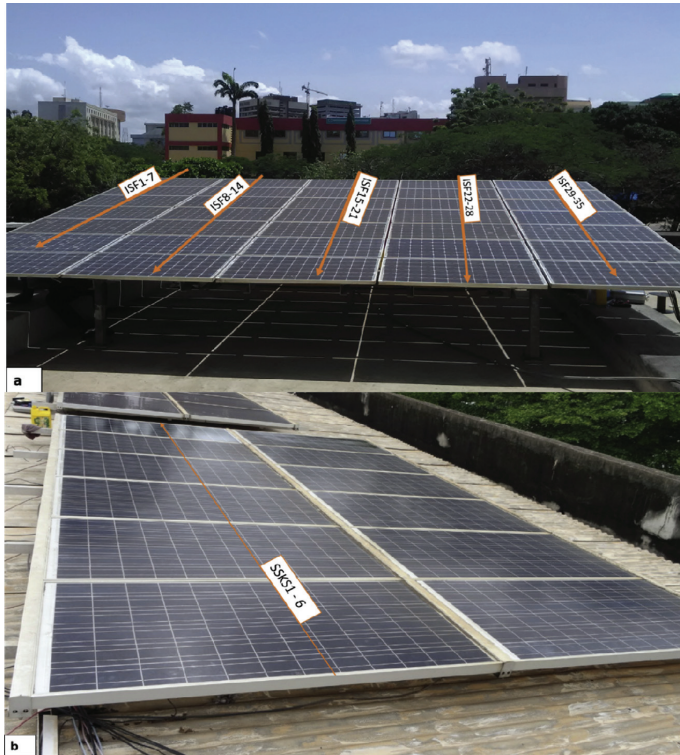
Fig. 2 – Pictures of installations: (a) MoEn grid-connected system and (b) KNUST grid-connected system.
