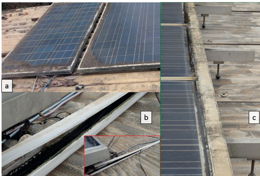
a) Low-tilt roofflushed modules with extensive soiling b) Cable ducts retaining water (with inset). c) Installation frame impeding water run-off.
