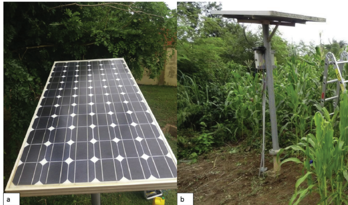
Fig. 4 – Water-pumping installations: (a) CWSA1 and (b) CWSA2.
