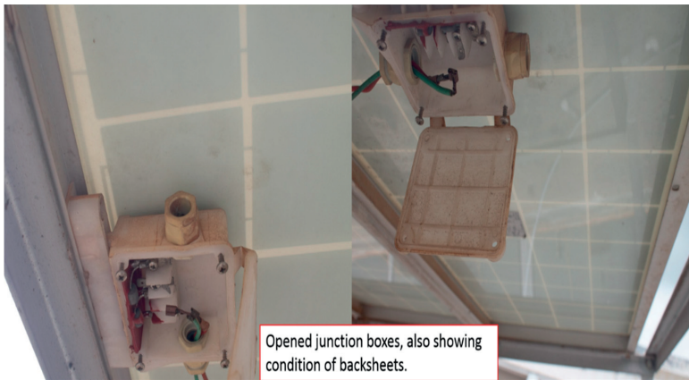
Figure 9. Junction box of modules, also showing backsheet.
