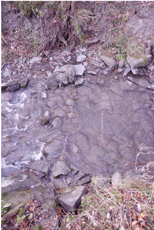
Figure 4: Antenna cable secured in the stream bed.
