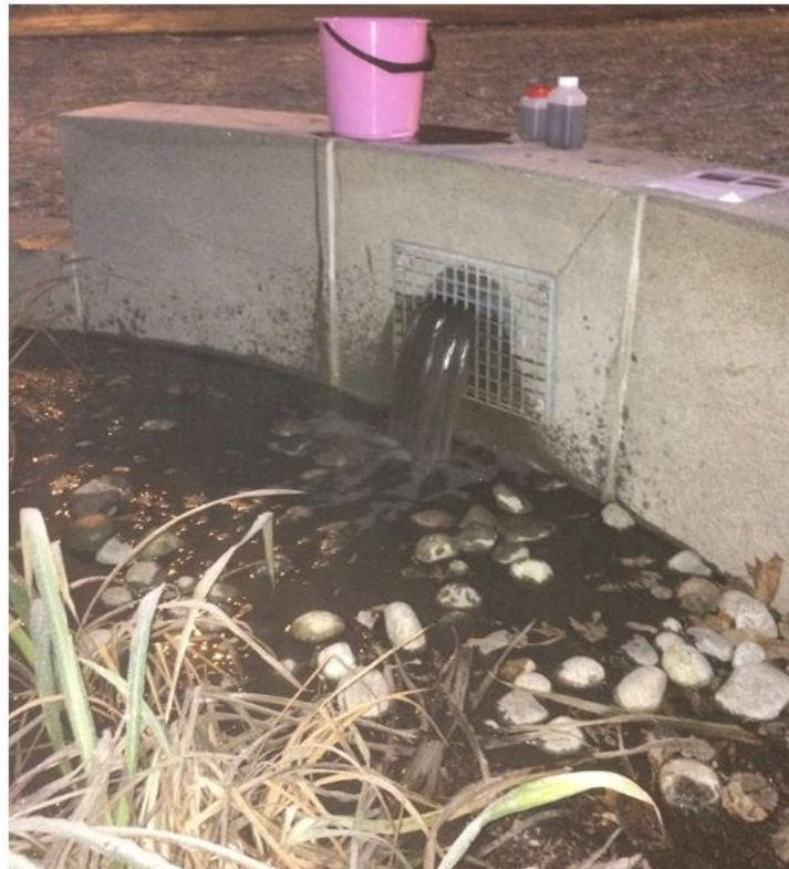
Figure 3.7: Treated wash water discharged from the sedimentation basin to the rain garden. Photo: Jon Petter Johnsen.
