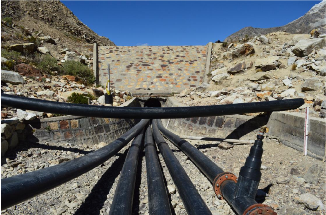
Figure 3.12: Four drainage pipes at Palcacocha. Adapted from Vilca (2016a).
