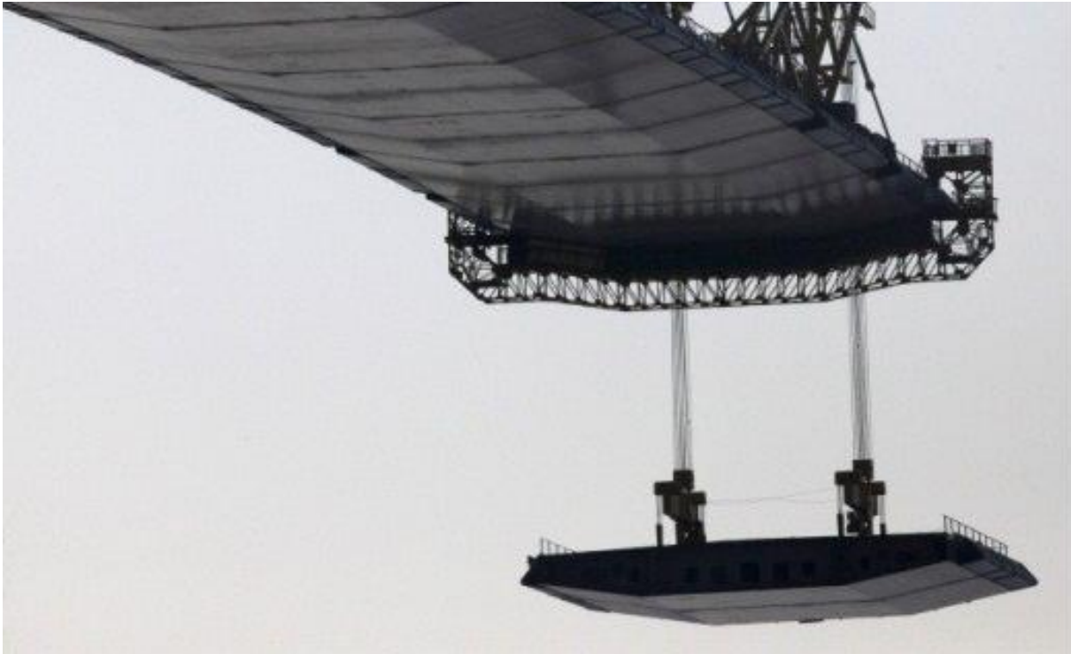
Figure 2.2: Illustration of bridge girder being connected. The picture is found in (Haque, 2015) and (Science, 2013)
