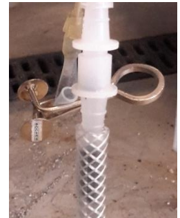
Figure 8.3-1 Clog in the filter inlet before the pump.
