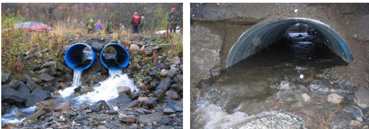
Culvert constructions at Bones; old (left) and new (right). New culvert construction facilitating the movement of organisms between the main river channel and its tributary (Hoseth 2017).
