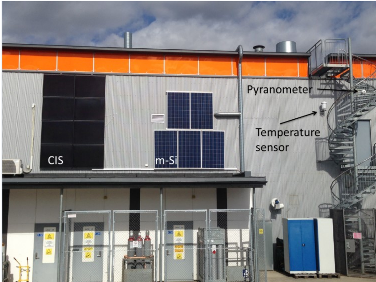
Figure 3.1: A picture of the test site, explaining where the two systems is mounted and where the pyranometer and temperature sensor is positioned.
