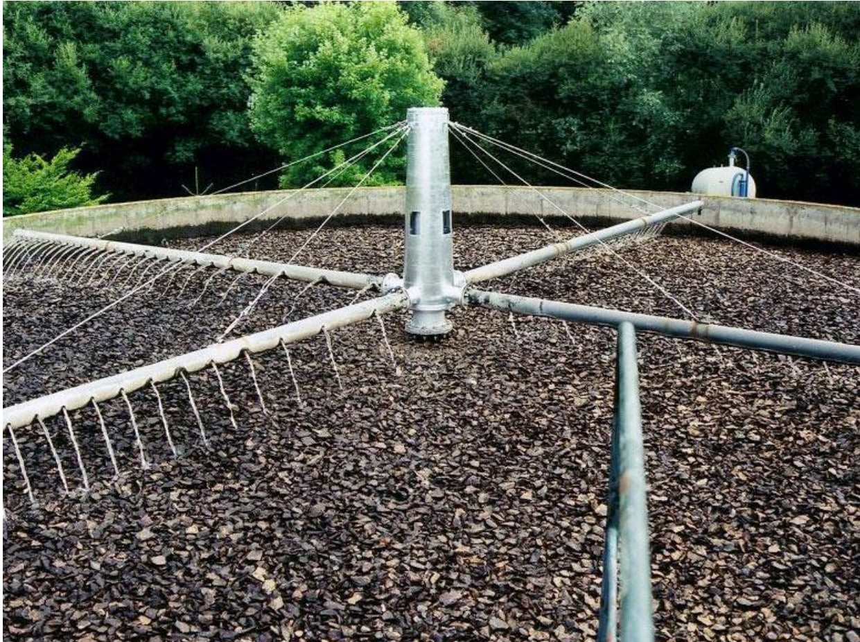
Figure 05: Bio-filter with nozzle for even distribution over the filter material. Picture is taken from (fbprocedes.com).
