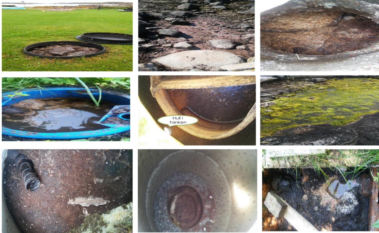
Figure 31: Mosaic picture of some septic tanks and their surroundings in Frøya. Some tanks have holes, the others are filled from sludge due to lack of proper pumping out of sludge and so on. Photo courtesy: Frøya Kommune.
