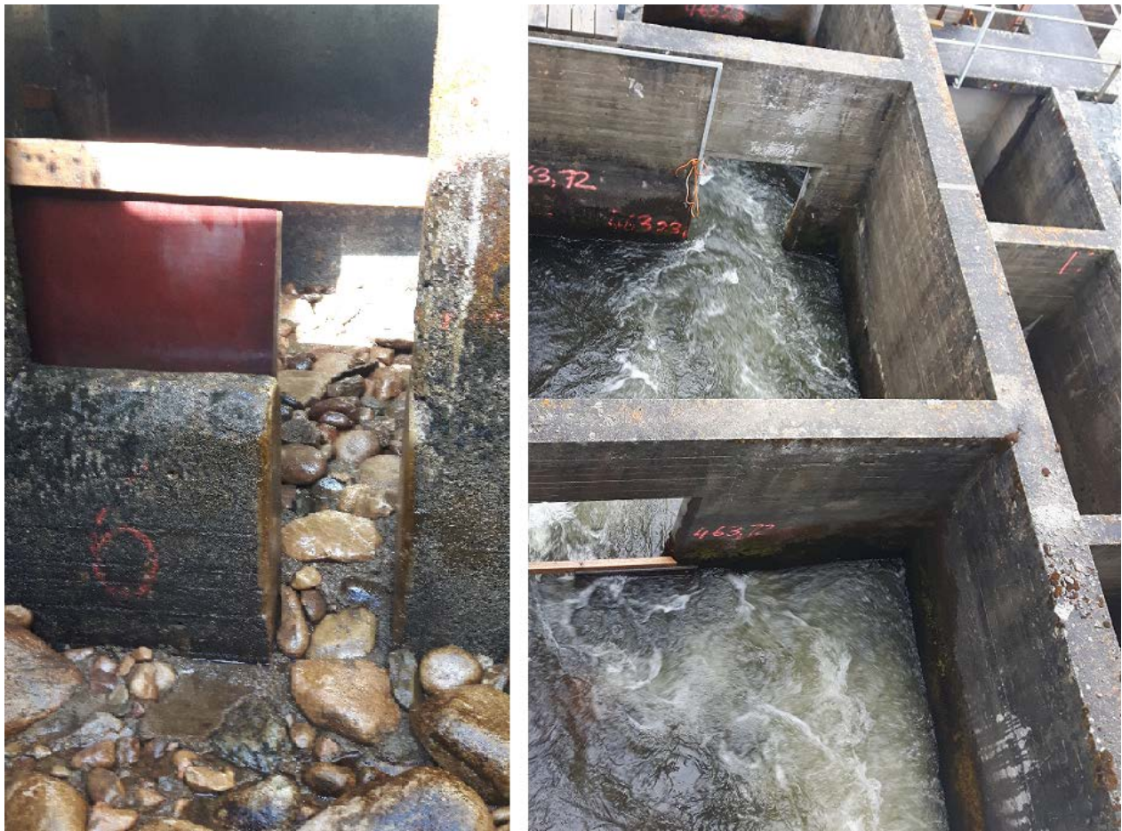
Figure 6 - Left: The new design with 30 cm wide slots and added substrate allow fish to swim along the bottom to ascend the fishway. Right: The picture is showing how it looks in two chambers when the fishway is in operation. Both pictures was taken during the excursion April 10 th , 2017.
