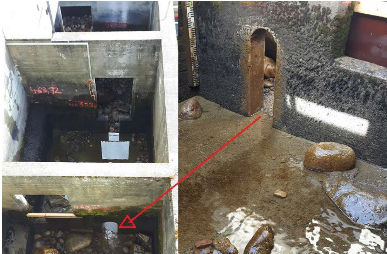
Figure 8 - Both pictures are taken after the reconstruction on the 10 th of April 2017, before deployment of the VAKI Riverwatcher. The red arrow illustrates where the right picture is taken relative to the left picture. Left: Chamber number 15, seen from above. Right: The exit of the same chamber. It is almost no added substrate in the bottom of this chamber because the VAKI Riverwatcher needs to be mounted in a stable position.
