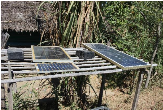
Figure 2.4: Solar PV panels used for lightning purposes
