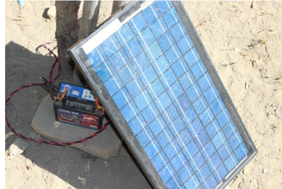
Figure 2.5: Solar PV panel in combination with battery
