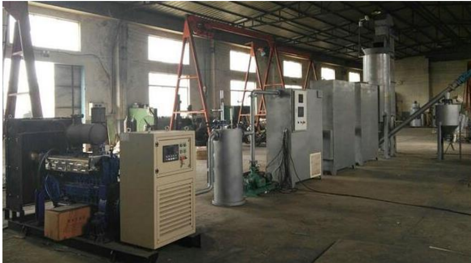
Figure 4.3: Bio Gasifier Power Plant (e-mail correspondence 2017)
