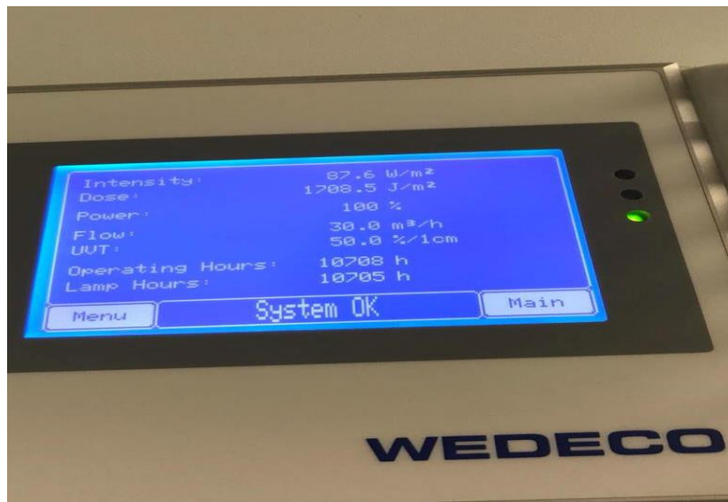
Figure 10: Screen of UV reactor (WEDECO BX80e FAN)
