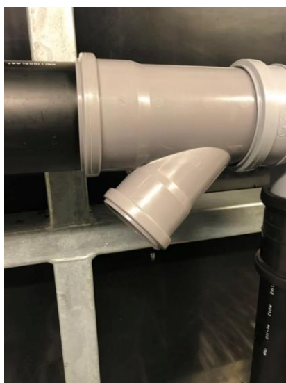
Figure 15: Outlet pipe of drum filter
