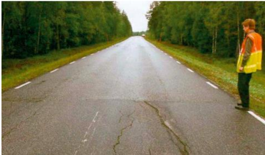
Figur 2-20: De langsgående sprekkene stopper der asfaltarmeringen starter [12]
