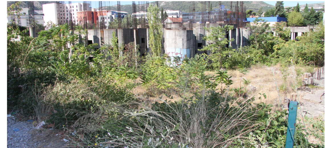
Figure 97: From the future sports-centre, one can view the north-eastern part of the plot which is currently overgrown and has a concrete-structure. (Brkan,2017)
