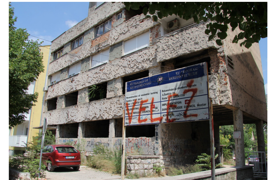
Figure 105: A destroyed apartment building on the Santic Street. (Brkan,2017)
