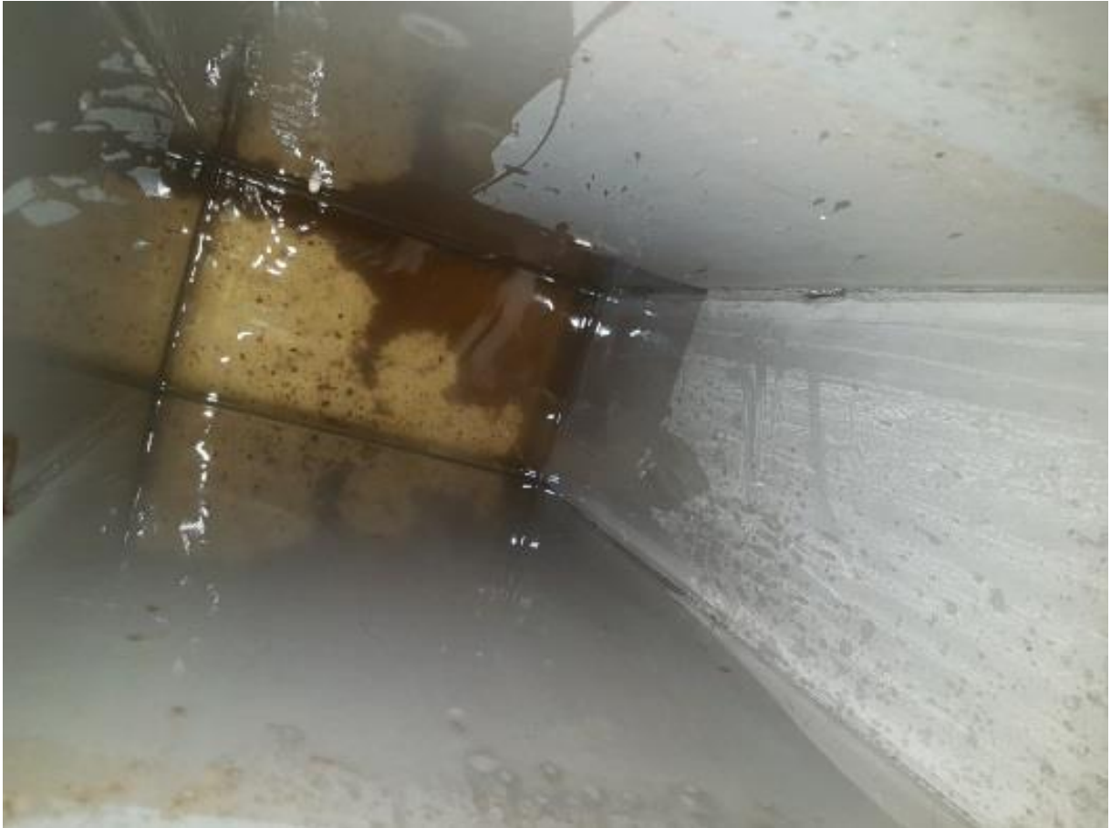
Figure 21: Sludge collection at the permeate tank
