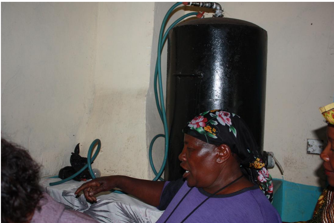
Photo 6: An ordinary LPG gas cylinder modified to store the excess biogas. Photo (Wamwea, 2010).
