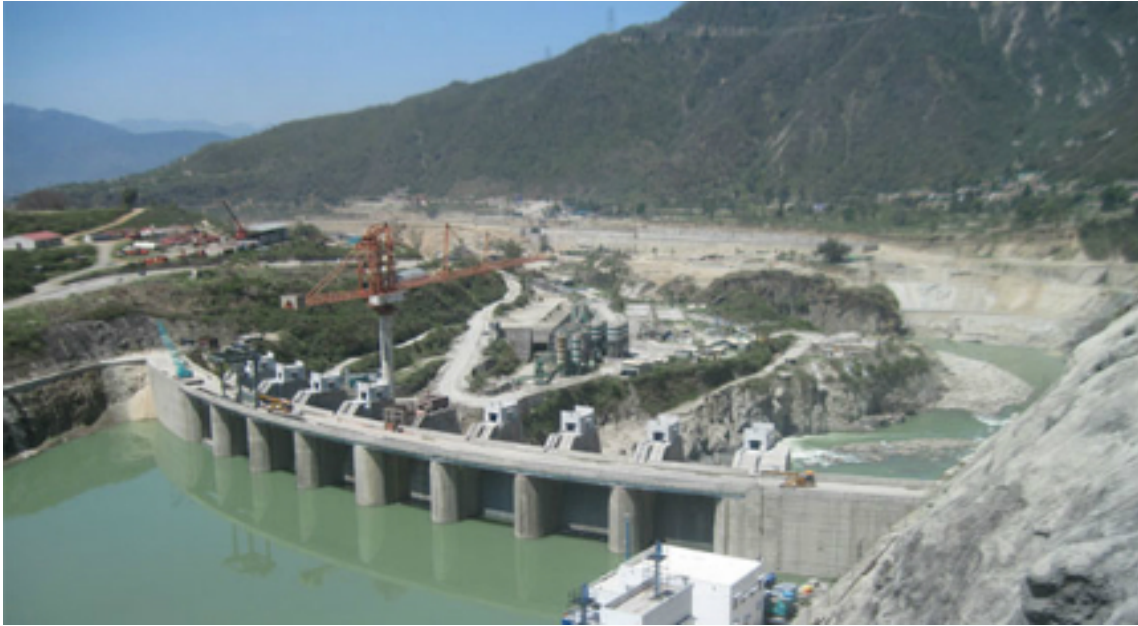
[Figure 5: A recently taken image of an under construction Hydropower plant at Alaknanda Hydroelectricity project, Uttarakhand, India; after building a water dam and storage the river water the downstream area dried out and looks like small desert, there is almost no trees and plants around a couples of kilometers after the construction of this dam completed]
