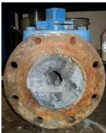
Figure 3 - Struvite deposit in pipeline 4
