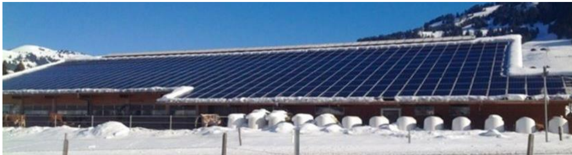
Figure 12. The HAIN system covering the complete area of a sloped roof.
