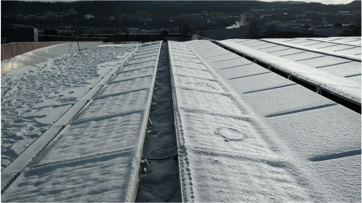
Figure 49. The photo shows the 2 strings subjected to current, with the untouched strings next to it on the right. The modules facing the wind(left) formed an ice cap, while the modules sheltered from the wind(right) did not.
