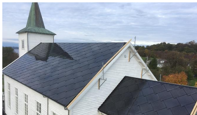
Figure 92. Strand Kirke in Rogaland has a coherent, frameless, integrated PV surface, favorable for sliding snow off the roof. (Enova 2016)
