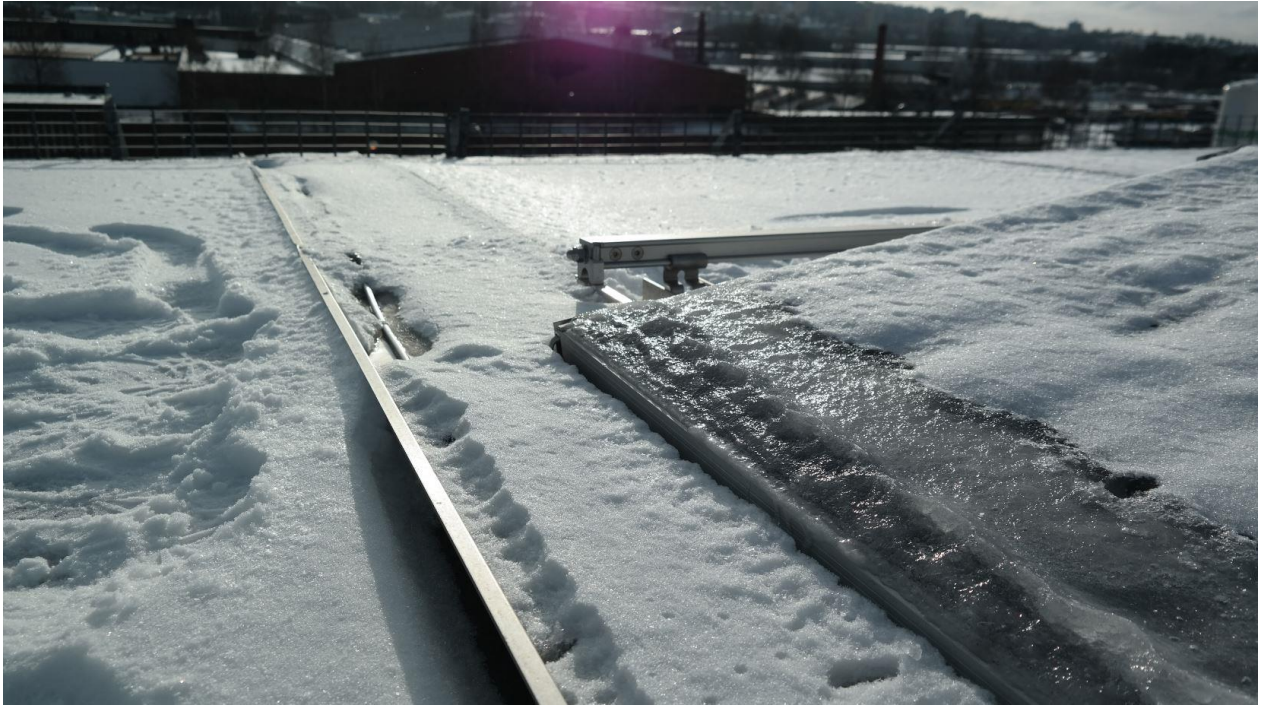
Figure 47. An ice cap forming at the lower edge of the modules facing the wind
