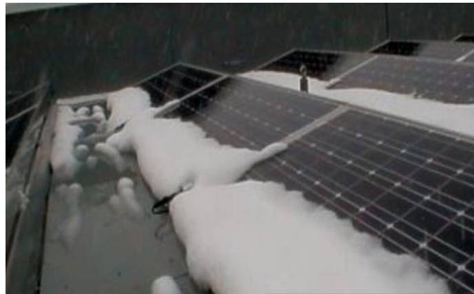
Figure 91. The HAIN system in progress. For this particular installation, the snow is only partially slid off the module, not optimal for enhanced solar gains. The installation then relies on the melting the rest of the snow to clear the module surface (KEI Solar 2017).
