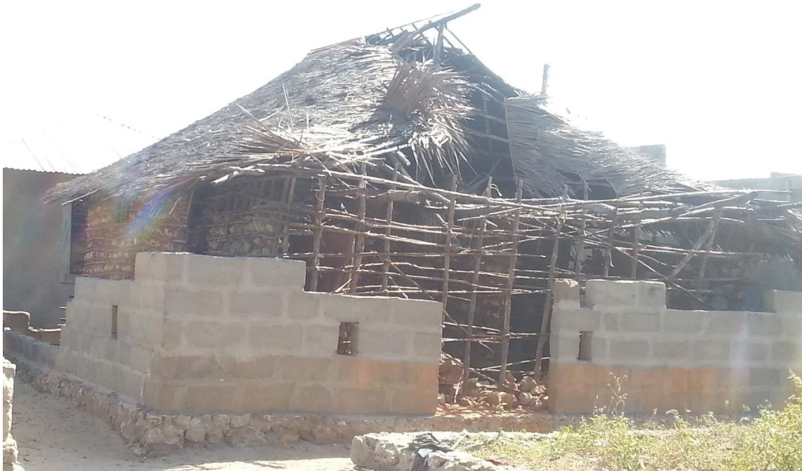
Figure 10. Mangrove poles and mud made walls on a house being replaced by concrete block walls at Vanga. Photo: Murungi, E.M. (2017, February 1).
