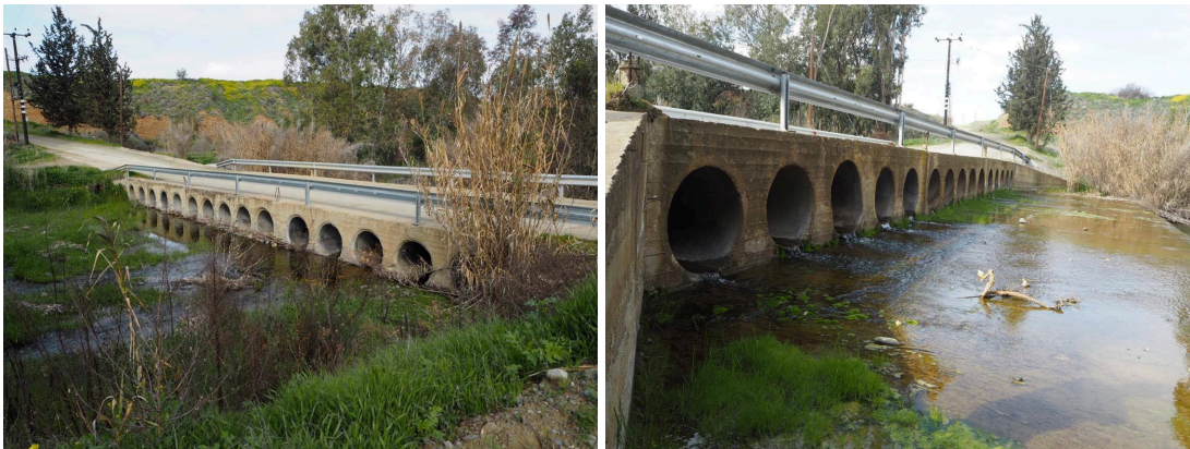
Figure 43: Bridges built with integrated culverts for water drainage in relation to road systems.
