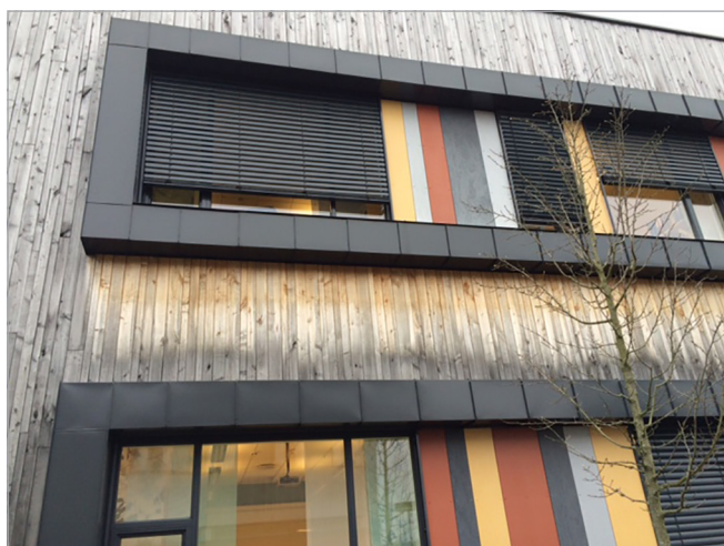
Figure 1. Unevenly weather-exposed wooden surface on a building façade, Aas, Norway.
