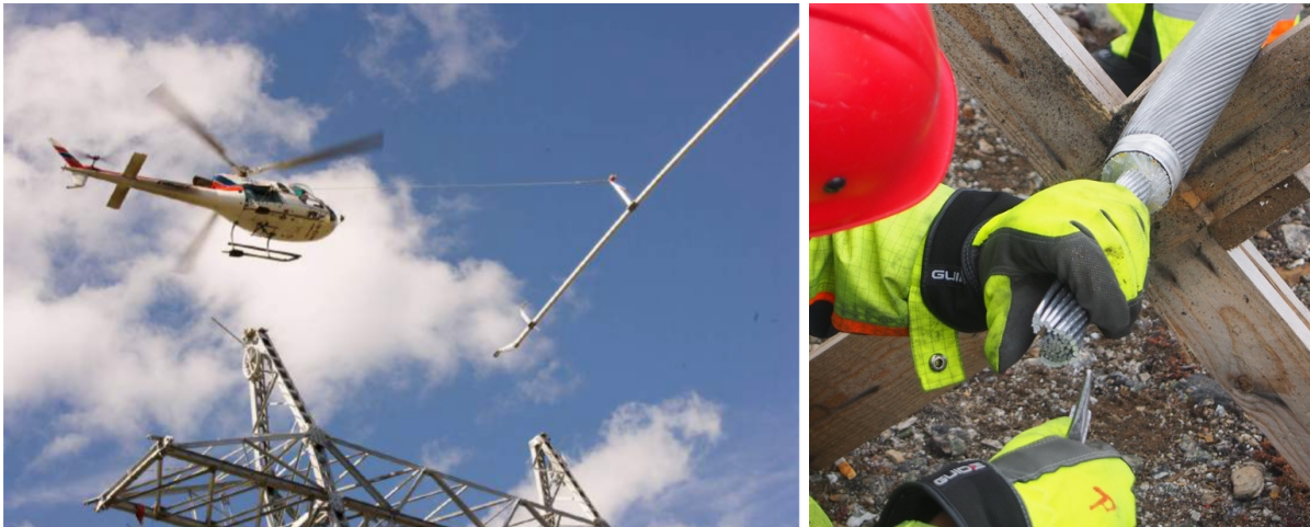
Figure 3.9: Left: Helicopter placing a pilot line in a tower using a needle. Photo from Statnett Right: Dismantling of thick cable so that a dead end clamp can be fastened. Mounting ring is fastened on the outer layer by explosives.
