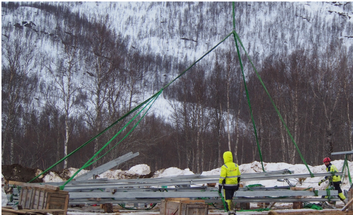
Figure 3.4: Tower-piece lifted from the top of another tower piece with the use of helicopter.
