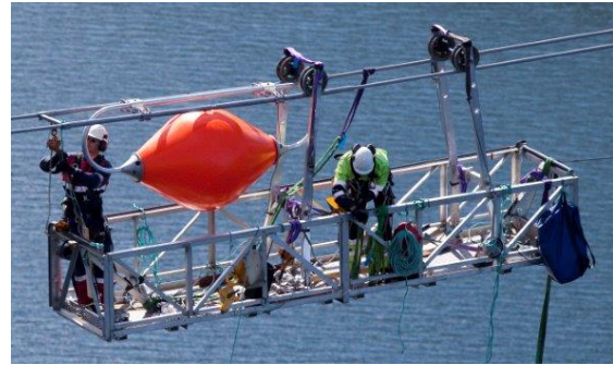
Figure 3.11: Crew in a trolley working on an aerial marker. Photo ©: Trond Isaksen, Statnett
