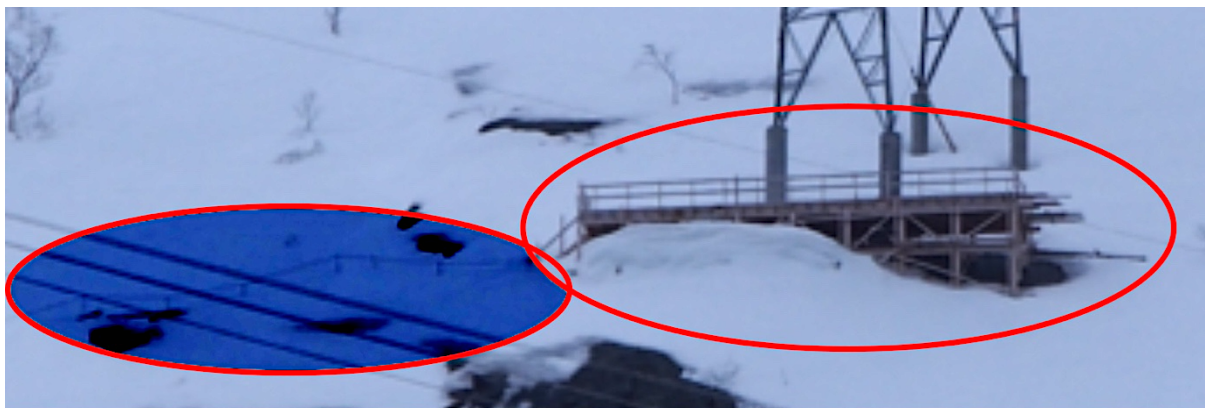
Figure 3.7: Iron path in the left blue circle (edited for higher contrast) and scaffolds in the right circle for construction of foundation. The concrete columns are also elevated on each leg to resist avalanches.
