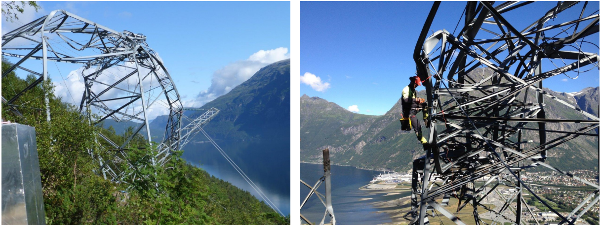
Figure 3.10: Left: Damaged tower. Photo by Egil Bjørgen © Statnett
