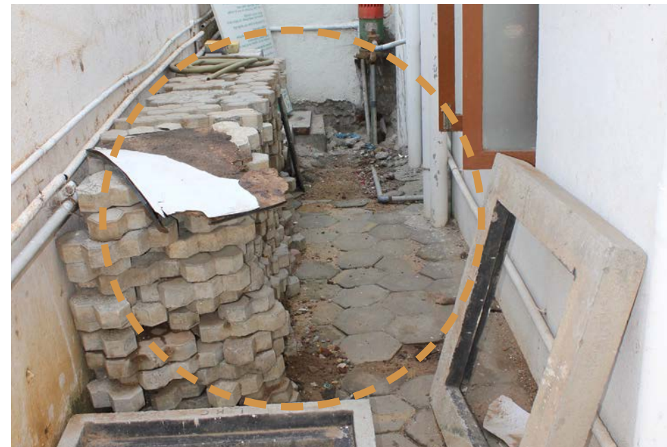
Garbage and building material lying around.
