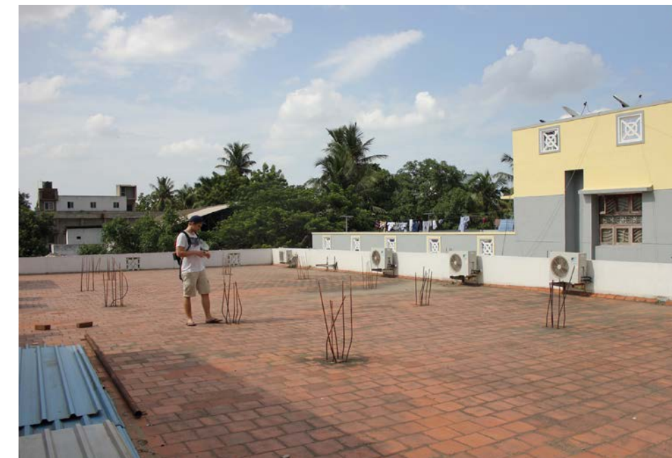
The roof terrace with dangerous rods sticking up.
