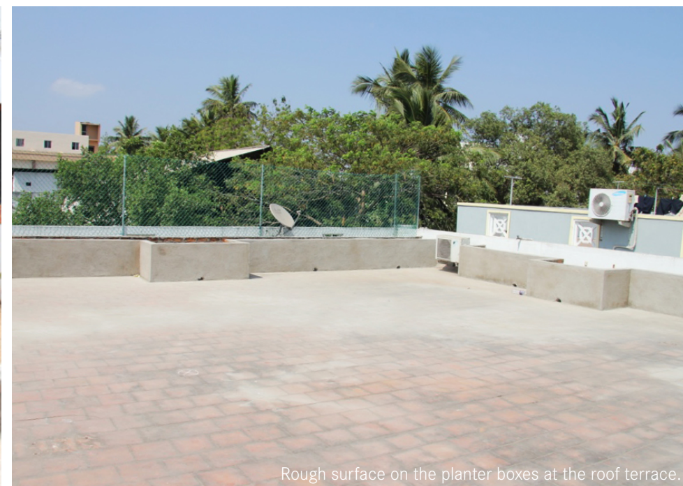
Rough surface on the planter boxes at the roof terrace.
