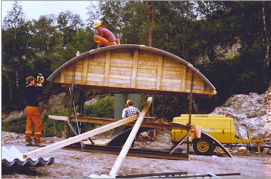
Figure 2.6. Template used to form the bedding into a desired curved form (Vaslestad 1985).
