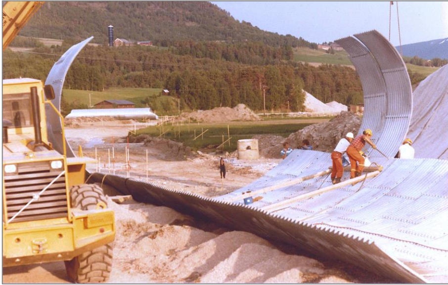
Figure 2.8. The side plates bolted together with the base plates 'in situ' (Vaslestad 1985).
